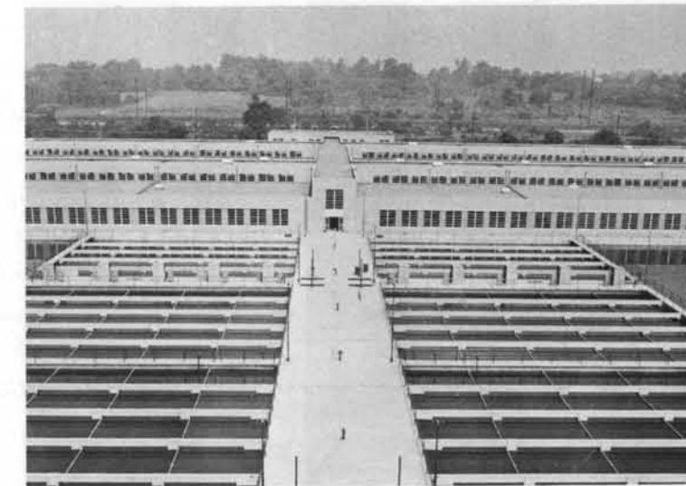
Treatment facilities: Water and chemicals are stirred in slow mixing basins (center) to form snowflake like "floc". Filter building (rear) houses rapid sand filters.
