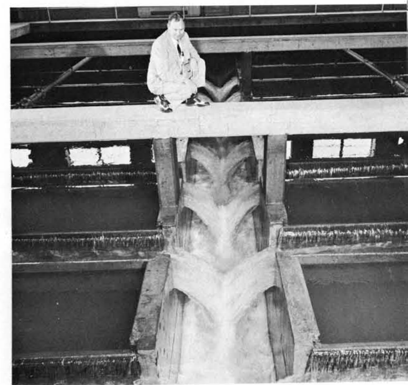
Washing: Rapid sand filters can be cleansed within a half-hour. Pure wash water is forced up through sand and gravel to carry away debris.
