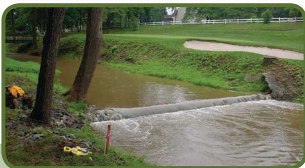
This small dam at the Brookside Country Club in Pottstown, Pennsylvania, was partially removed to allow fish passage as part of a stream-restoration project funded by the Schuylkill Watershed Initiative Grant.
