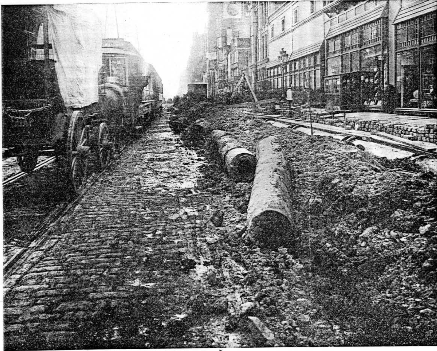
THEN AND NOW—Old wooden pipes recently removed from Market street near City Hall; these pipes were laid in 1801. Prior to 1817 all water mains in Philadelphia were made of wood, and as late as 1845 there were still in use 45½ miles of wooden main, although the City had then a population of nearly half a million.
