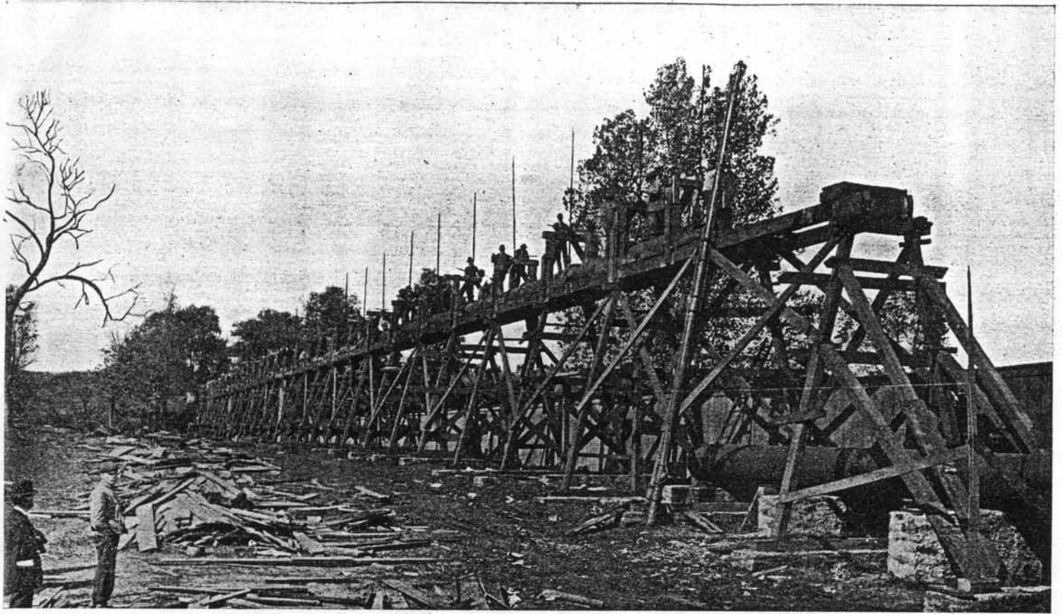
DIFFICULT WORK OF LOWERING 1,200 FEET OF THIRTY-INCH PIPE a distance of twenty feet. This work was made necessary to allow grade of new Northeast Boulevard to pass above existing water mains.
