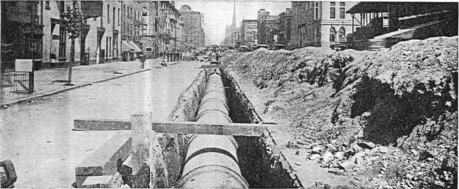
LAYING A FORTY-EIGHT-INCH WATER MAIN IN BROAD STREET, showing necessary disturbances of traffic.
