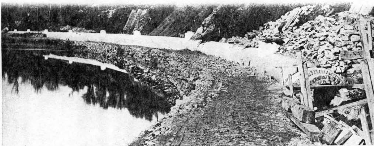
SHAWMONT INTERCEPTING SEWER, about three-fourths of a mile in length, serving Roxborough Filter Beds and environs, intercepting sewage from the Schuylkill River.
