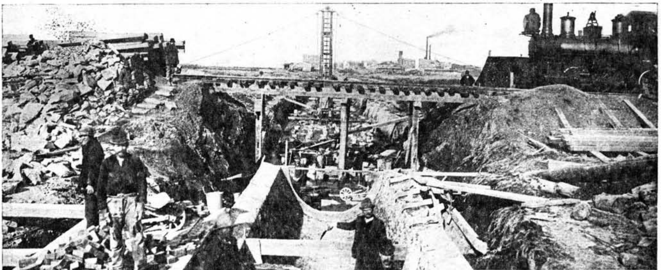
OUTFALL SECTION ON ONTARIO STREET SEWER, showing cradle resting on pile foundation. This sewer is two and one-quarter miles in length, eight feet in diameter and built of brick. It empties into the Delaware River, serving Ontario and Jasper, Delaware River to Sedgley Avenue.
