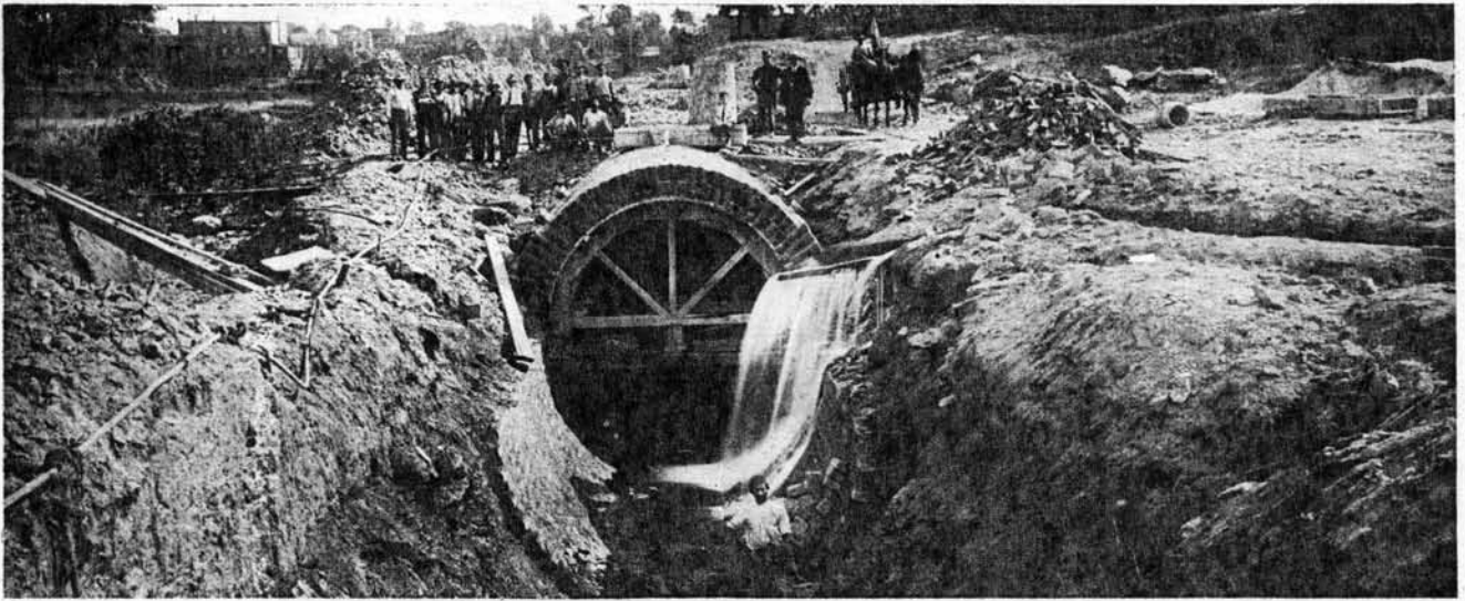
GENERAL VIEW DURING CONSTRUCTION OF ROCK RUN SEWER. This sewer is one mile in length, 12 feet in diameter. The Rock Run system of sewers has its mouth at Tacony Creek at the Boulevard and continues northwest to City Line, serving a district of 1,724 acres.
