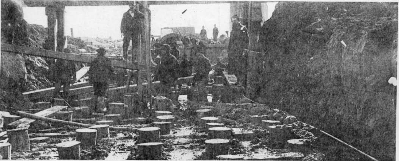
OUTFALL SECTION ONTARIO STREET SEWER, showing pile foundation, a feature in sewer construction involving considerable expense and causing delay.
