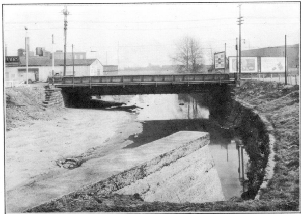
A- LOOKING DOWNSTREAM AT FRANKFORD AVENUE BRIDGE. SEDIMENT DEPOSITS RESTRICT WATERWAY OPENING
