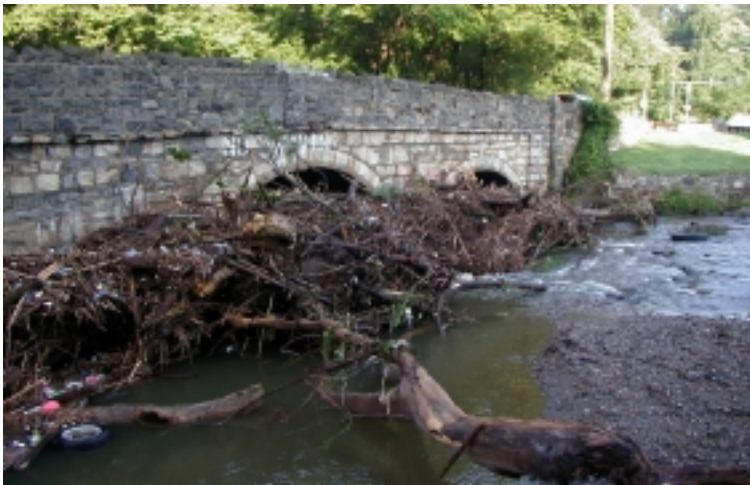
Adams Avenue at Crescentville Road following the August 1, 2004 storm
