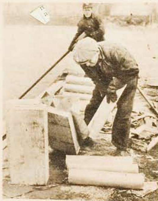
Workmen carefully unpack dynamite cartridges. For the blast, 600 25-pounders were packed in 113 holes in the river bottom.
