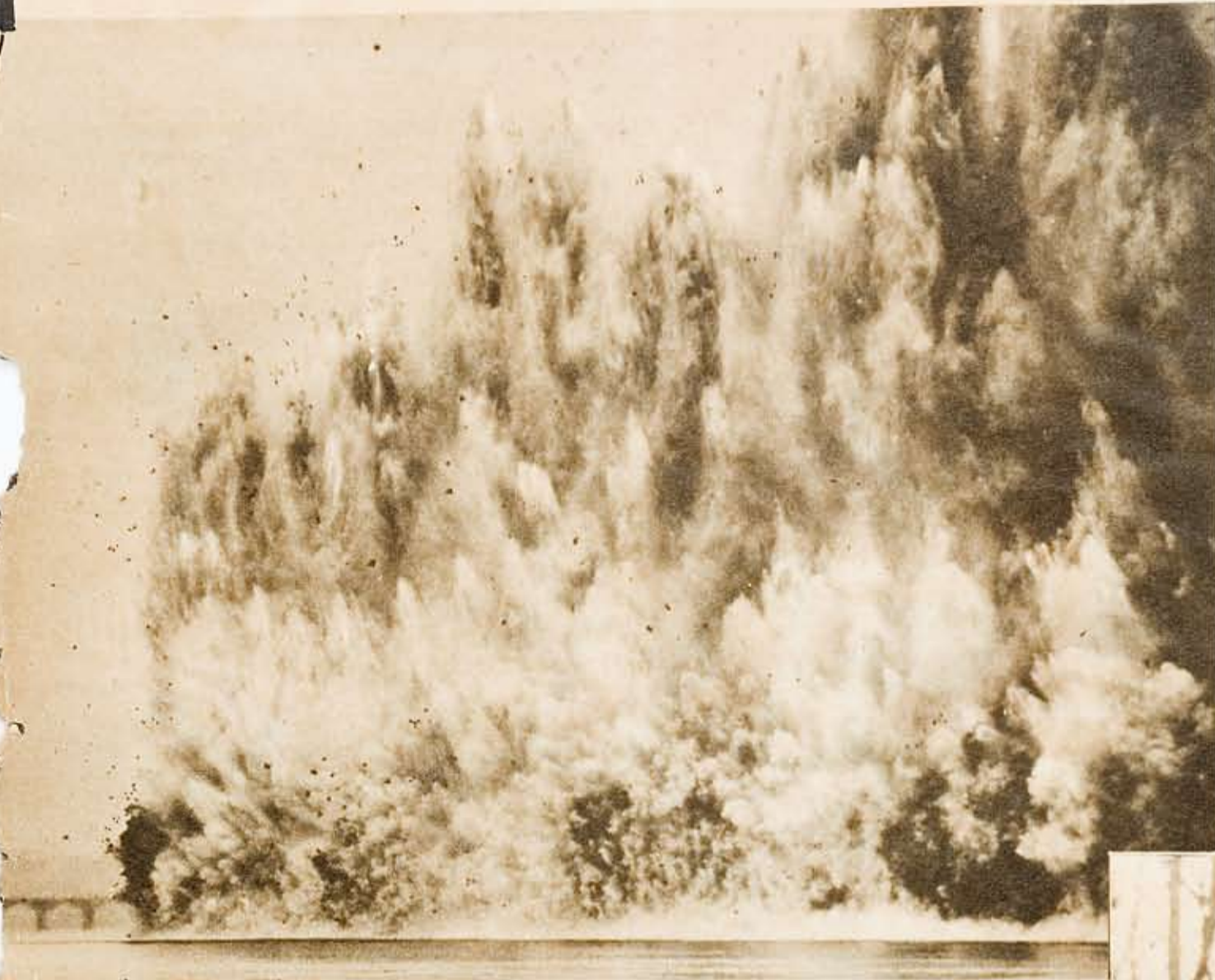
← In the biggest explosion yet set off in construction of the East-West pipeline (left), 15,000 pounds of dynamite hurled tons of bed rock, mud and water skyward.
