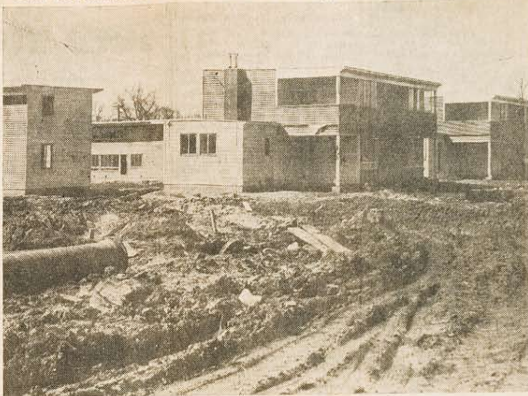
Part of the Pennypack Woods defense housing development which private builders say violates city building code. The buildings, of frame, are called "fire traps. The structure in middle is for four families
