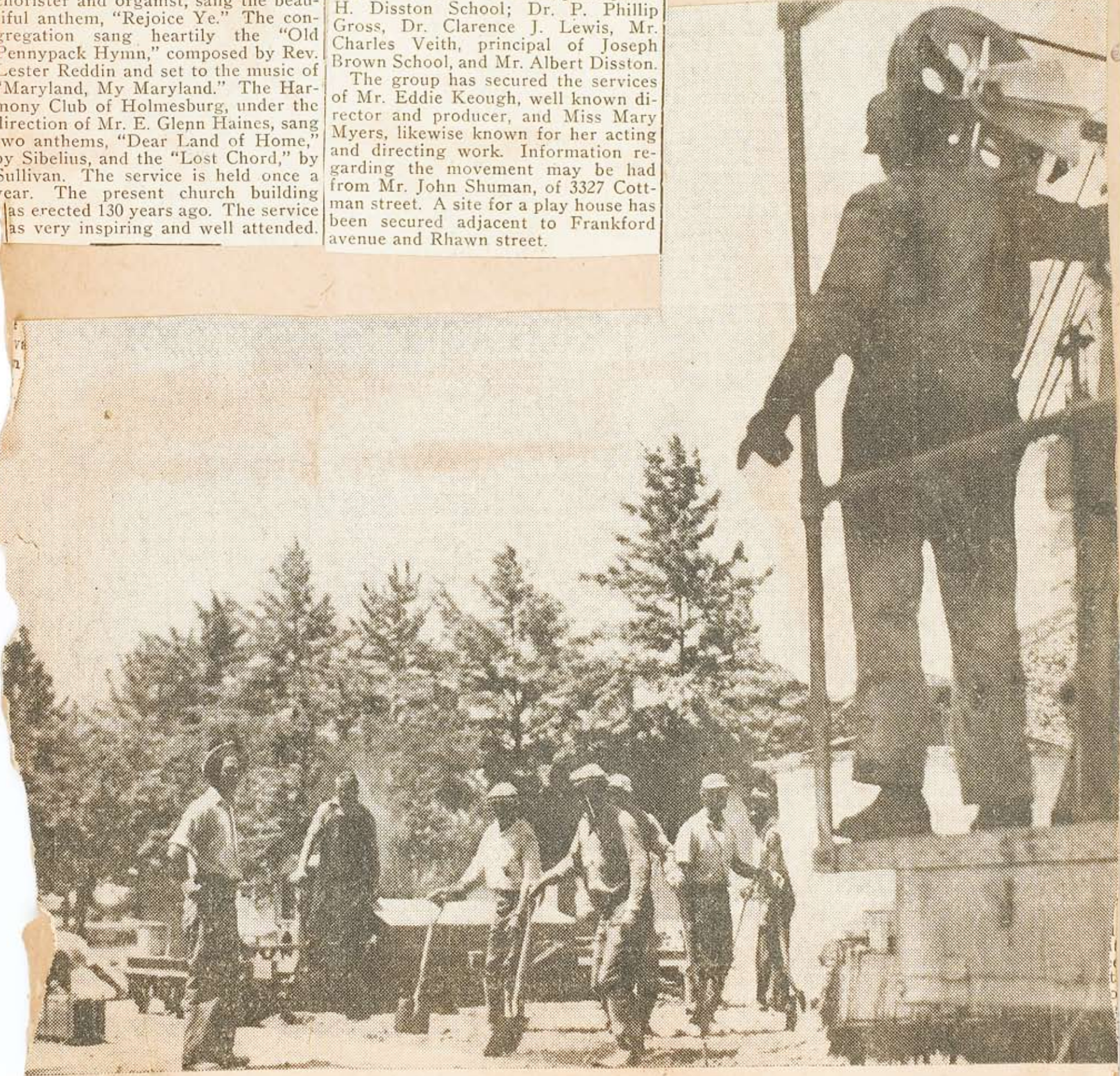
NG the concrete is also done by the mixer, but workmen spread it with their shovels and the
