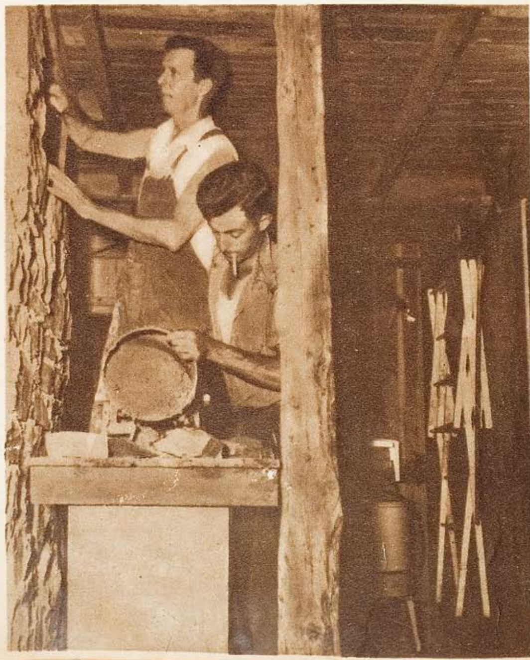
→ Chimney pointing is not the occupation of these workmen, but in Point Pleasant the jack-of-all-trades is everywhere. This odd job of masonry is being performed expertly by a foundry foreman and a telephone company employee.
