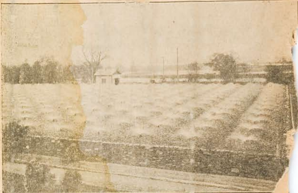
This Photograph Shows the trickling filters in the foreground, and in the background is the plant for chemical treatment of the sewage to purify it.
