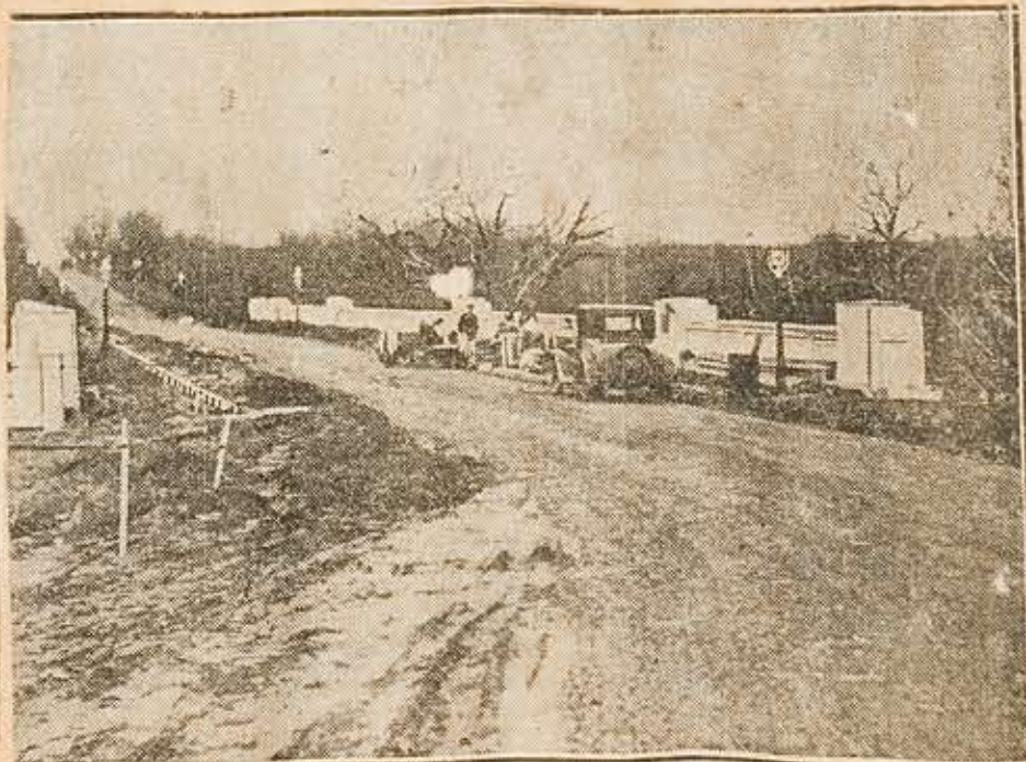
View of Rhawn Street at the East Bridge—The surfacing of the roadway is completed, except for the clean-up work. The West span is about six hundred yards distant from the East bridge, which is at the crest of the hill at upper left in picture. The diagram shows the location of the spans and the section of the city which they connect directly.
