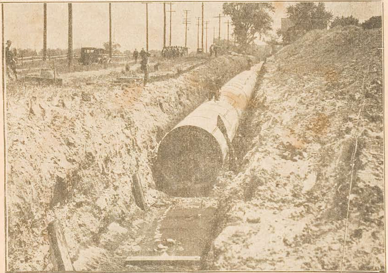
How the "Big Ditch" in the Northeast Looks—The pipes are placed so that the top of the main is four feet below the street surface. An army of mechanics, laborers, steam shovels and traveling cranes is employed on the big project. Work began April 1, and about one-seventh of the main has been laid. A section of the ditch immediately north of the Pennypack creek is shown.
