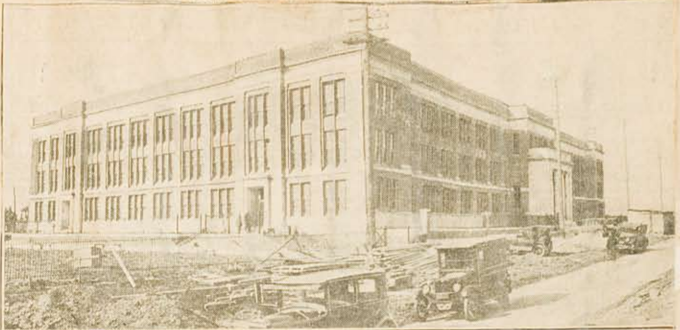
Woodrow Wilson Public School Nearing Completion, at Cottman and Loretta sts., upper Frankford. The Crossan Ordinance calls for the widening of Cottman st., shown in picture, from Oxford av. to Castor rd., a distance of about one and a half miles. This and other street improvements will give better bus access to the Wilson school for Burholme and Fox Chase children.
